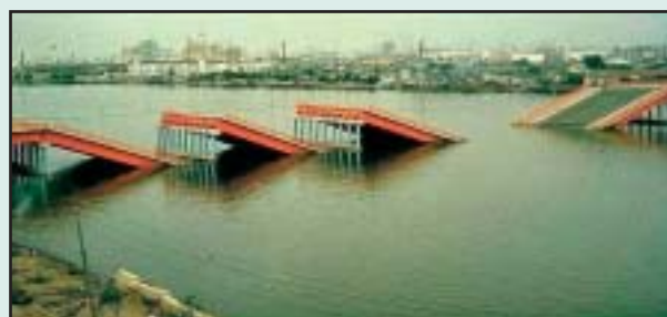
c) Failure of Showa bridge due to lateral spreading
